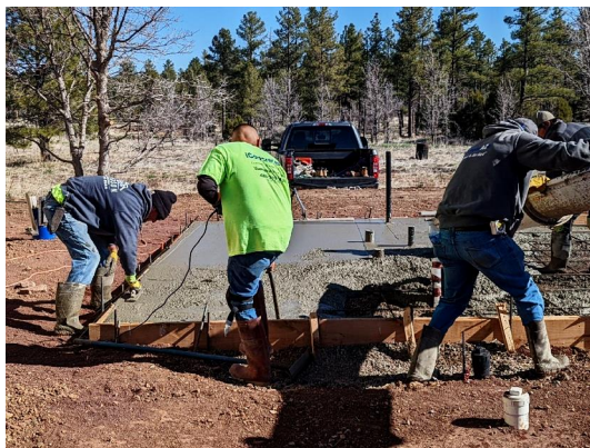
A crew from iConcrete led by Bruce Kremins pours tons of concrete to form the pad for our new food prep
