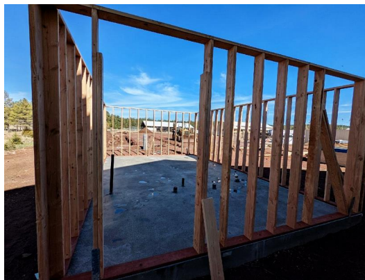
building. One day later, the 2x6 wood studs go up for the walls... finally, construction progress!
